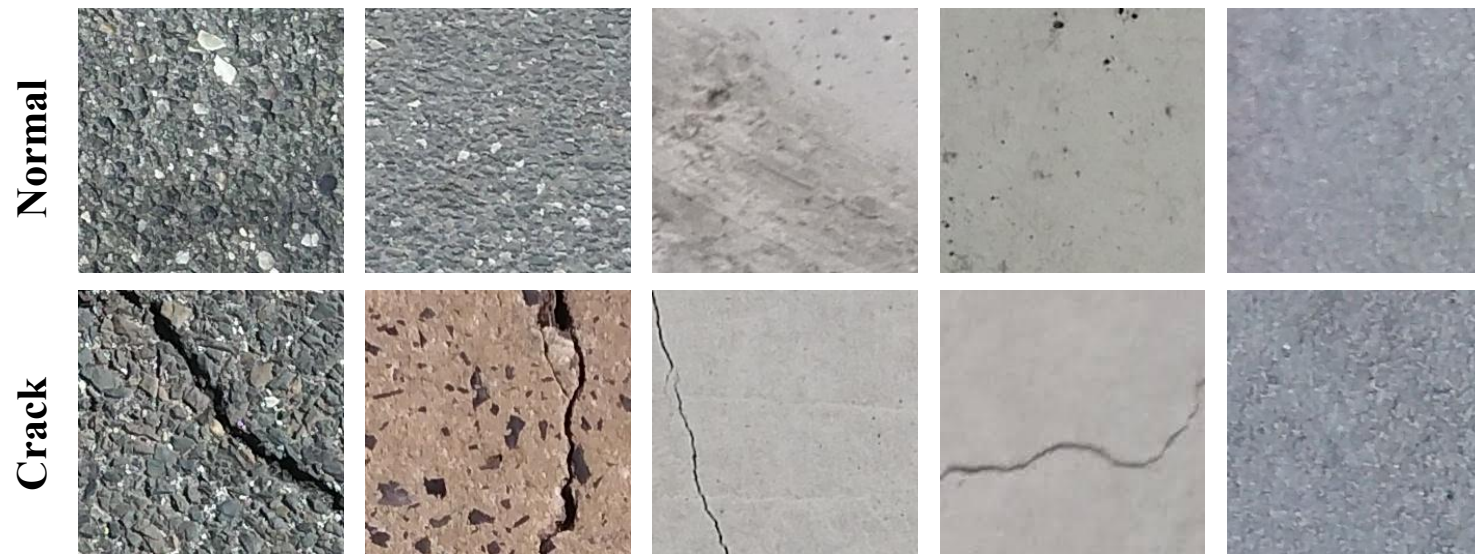
[Figure 1] Comparison of normal and crack images
